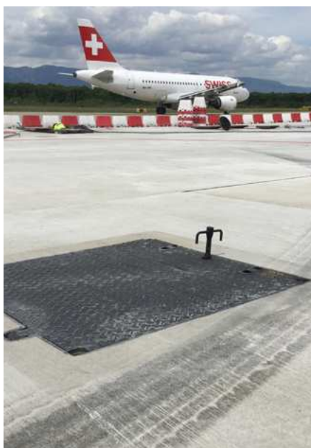
Geneva International Airport Switzerland Electrical network
