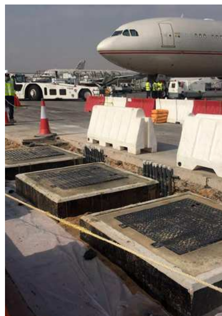
Abu Dhabi International Airport United Arab Emirates AGL network
